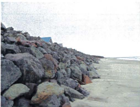
Photo 1. Looking south at the rock revetment at the Shoreline RV Park located about 900 feet north of the Pine Beach subdivision.
