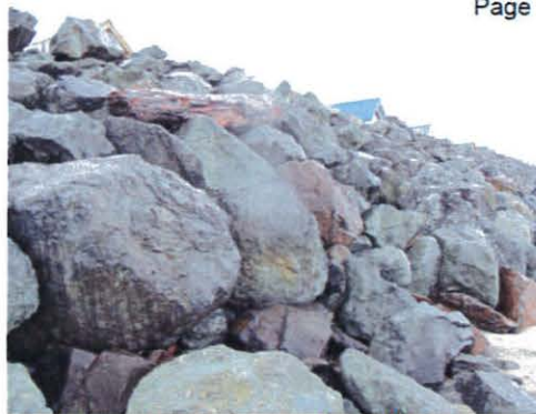
Photo 2. Close-up of rock revetment at the Shoreline RV Park located about 900 feet north of the Pine Beach subdivision.
