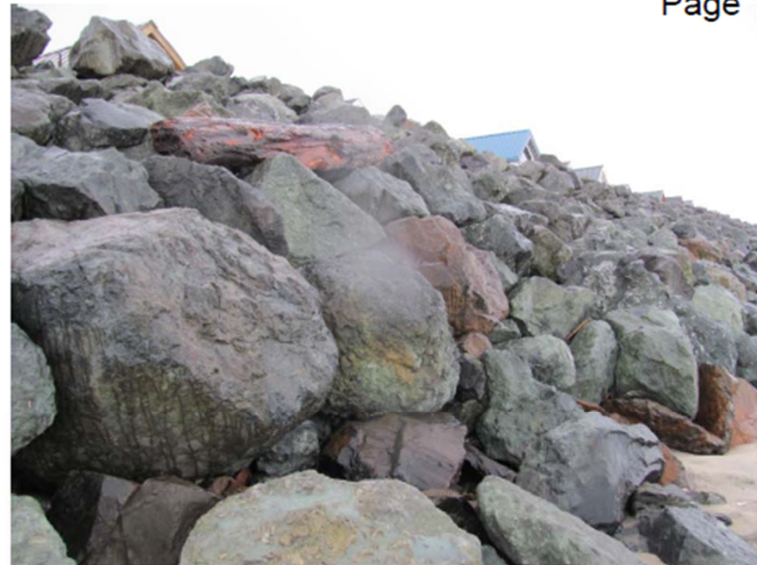
Photo 2. Close-up of rock revetment at the Shoreline RV Park located about 900 feet north of the Pine Beach subdivision.
