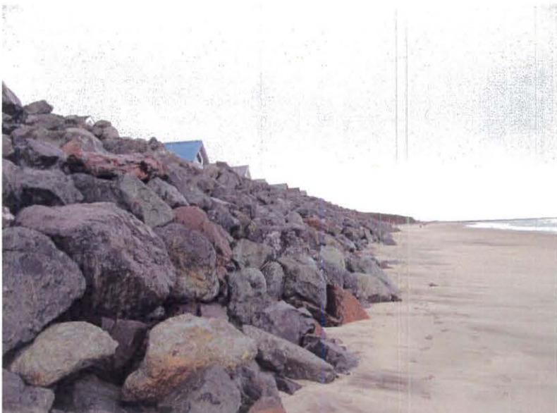
Photo 1. Looking south at the rock revetment at the Shoreline RV Park located about 900 feet north of the Pine Beach subdivision.
