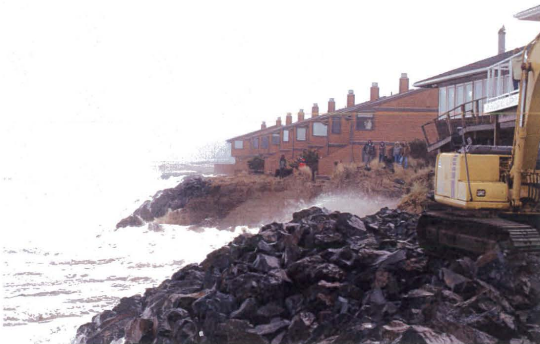
Figure 18. Erosion during a storm on January 5, 2008, eventually caused part of a riprap wall to fail in the town of Neskowin. (Photo courtesy of the The Breakers Condominiums, Neskowin, Oregon.)
