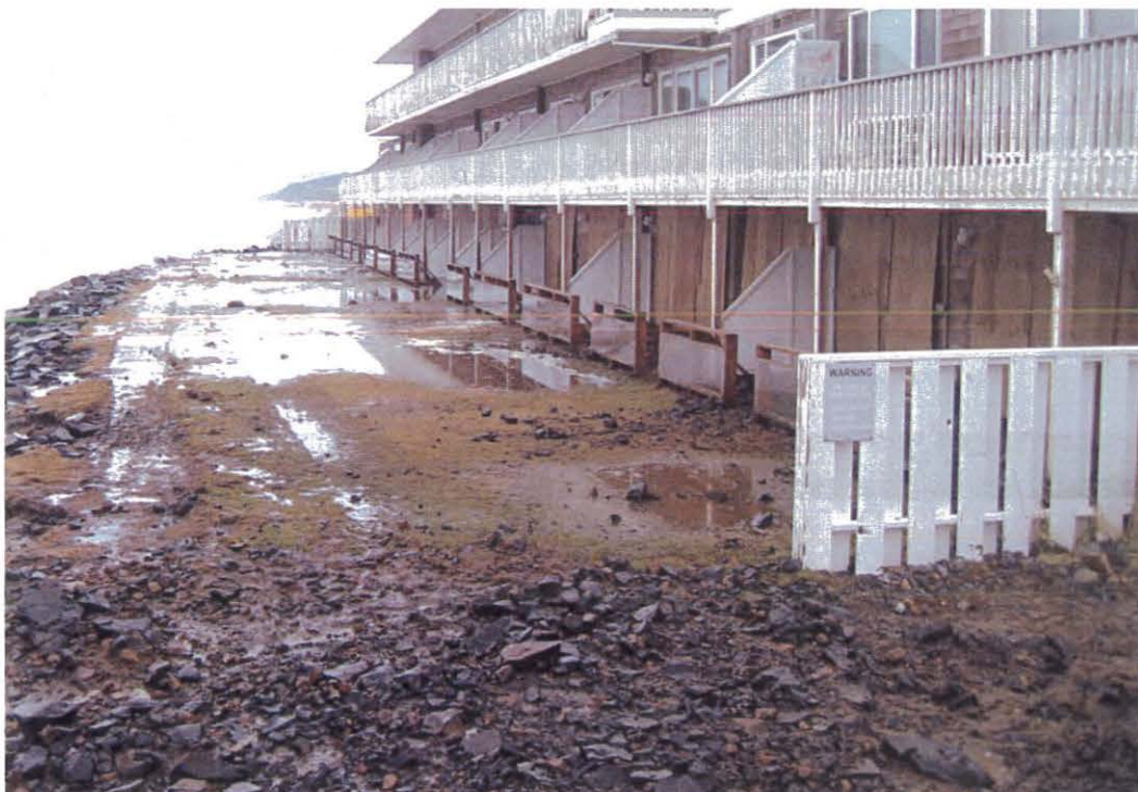
Figure 20. Overtopping of waves during the January 5, 2008, storm caused flooding and damage to ground floor condominium units located in Neskowin. Note that the crest elevation of the graded dune is 8 m (26 ft), while the condominium units are located approximately 6 to 10 m (20 to 30 ft) from the top of the riprap revetment. (Photo taken on January 9 at high tide.)
