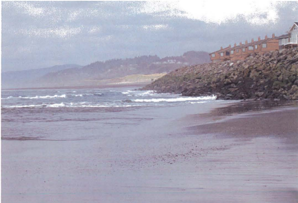
Figure 19. Development of a rip embayment north of Proposal Rock in Neskowin removed much of the fronting beach that would otherwise have protected the riprap structure shown above. Extreme lowering of the beach elevation means that the structure is being impacted by ocean waves at all tidal elevations. (Photo taken at low tide by J. C. Allan on April 15, 2008.)
