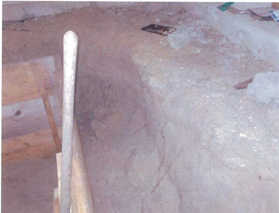
Photo 7 – View of the sand exposed in the crawlspace excavation.
