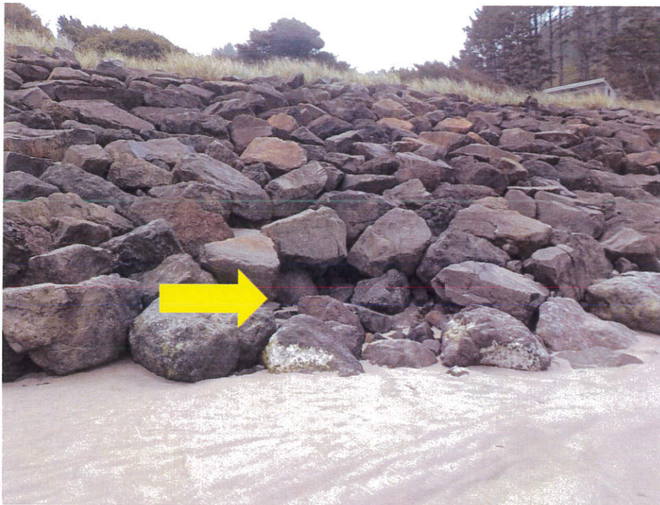
Photo 6 – View of the riprap revetment at the base of the slope immediately west of the site. Yellow arrow indicates where larger armor stone has become displaced and the revetment is damaged.
