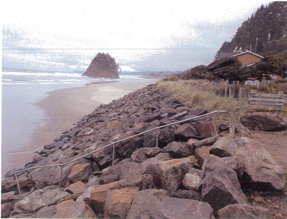
Photo 5 – Northerly view of the revetment, beach access stairs, and Neskowin Beach from just south of the site. Note the continuous riprap revetment along the dune slope.
