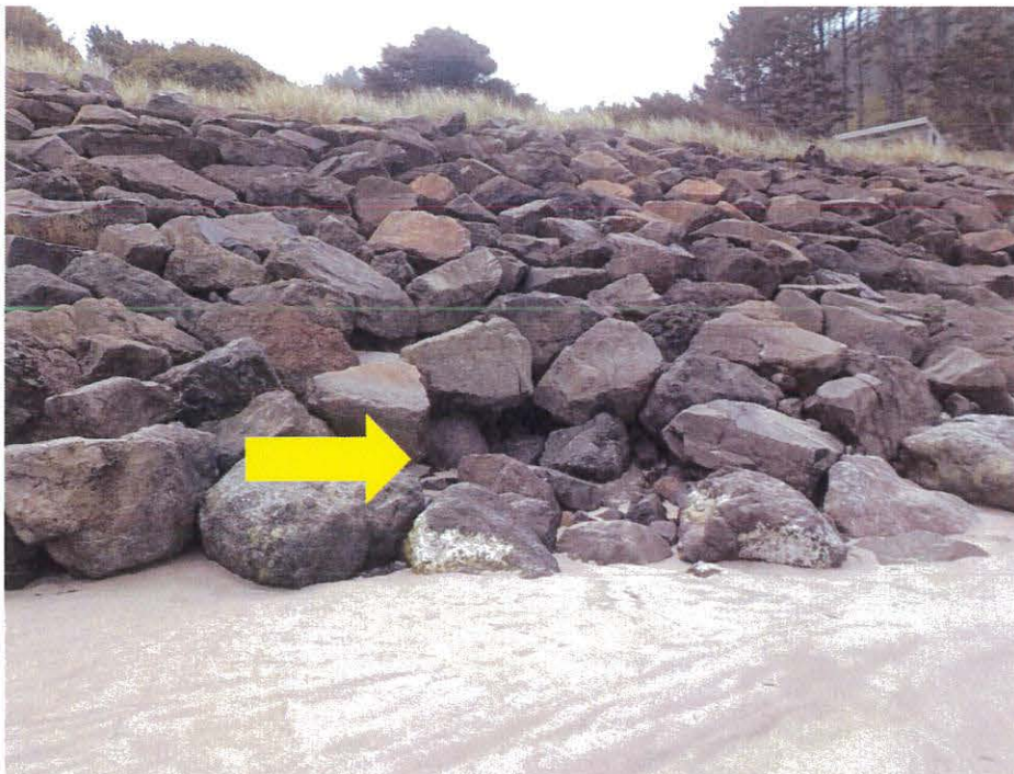
Photo 6 – View of the riprap revetment at the base of the slope immediately west of the site. Yellow arrow indicates where larger armor stone has become displaced and the revetment is damaged.
