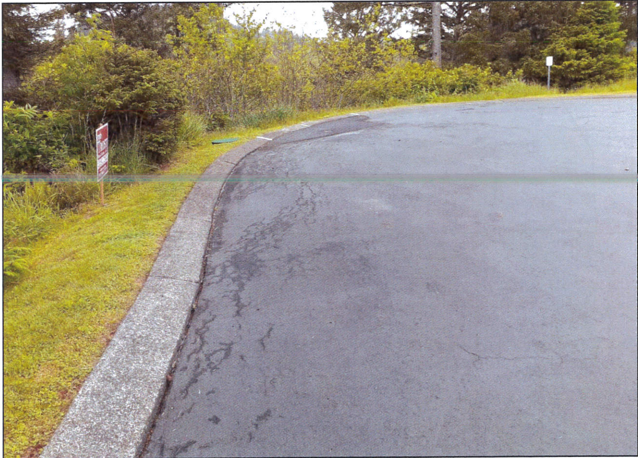
Photo 2 – View to east at north edge of Haystack Drive cul-de-sac. Lot 2900 is off left side of photo.
