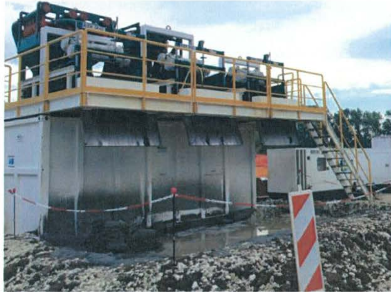
Figure 2. Example of a Drilling Fluid Mixing & Recycling Unit
