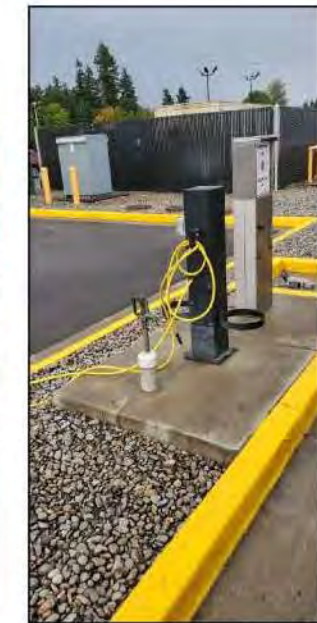
Pay station with water hose and electrical outlet
