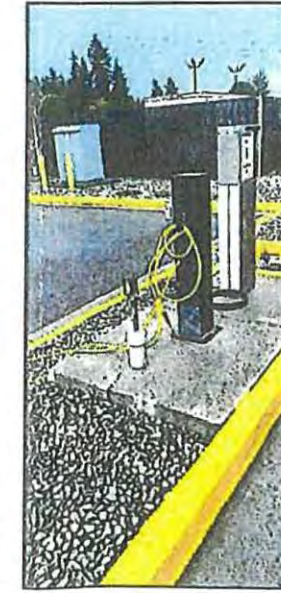
Pay station with water hose and electrical outlet
