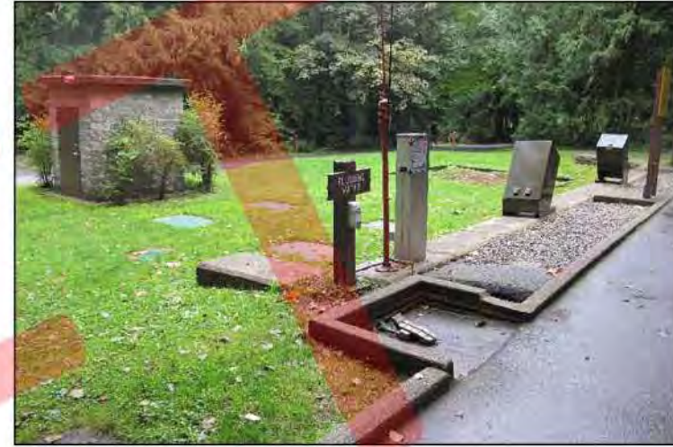
Typical pedestal location
