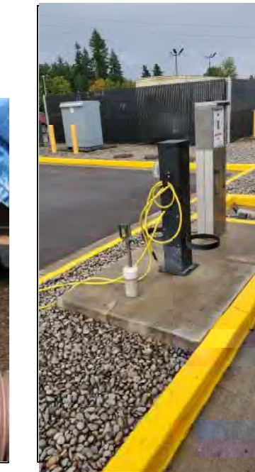
Pay station with water hose and electrical outlet
