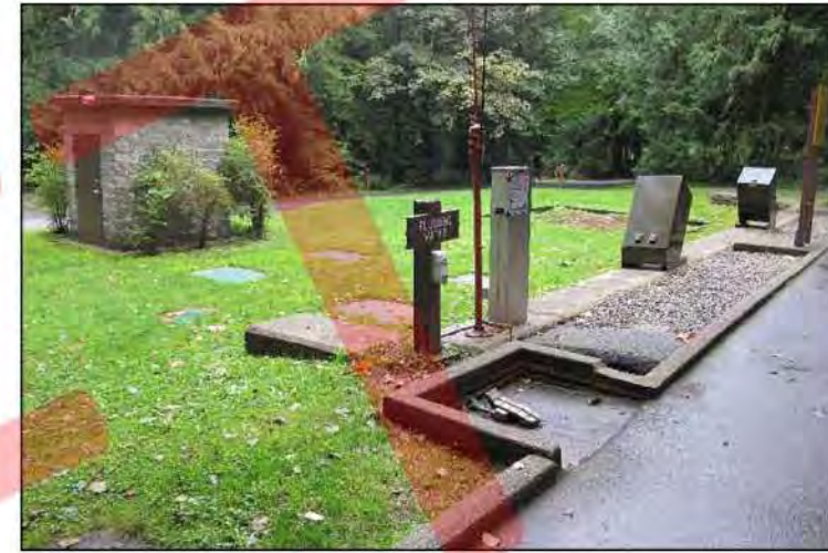
Typical pedestal location
