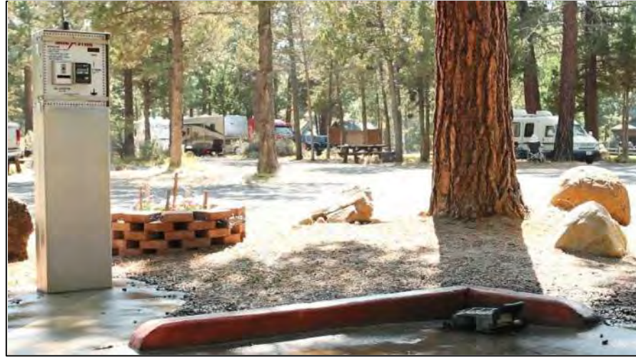
Typical Sanistar paystation location
