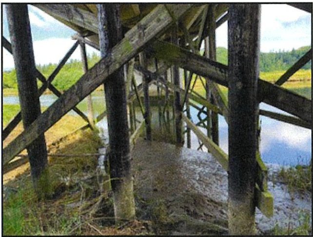
Photo shows the timber trestle substructure extending into the Tillamook River. Here, three piles will be repaired within Bents 6 and 8.
