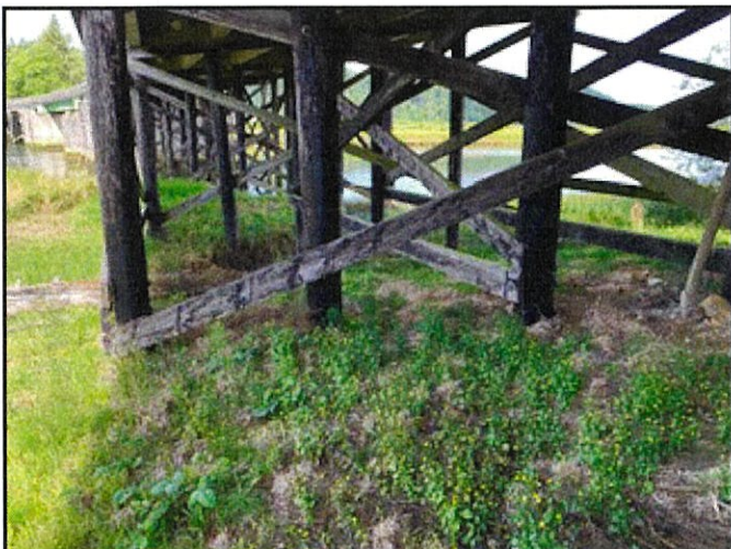
Photo shows the timber trestle substructure from the bridge abutment. Here, three piles will be repaired within Bents 14, 15, & 16. In total, 6 piles will be repaired.
