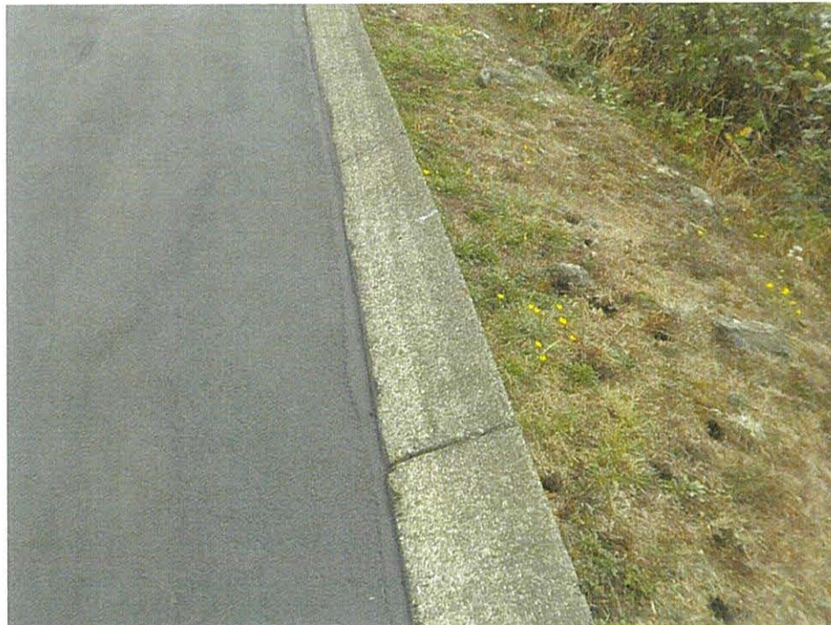
Photo 16 – View of the recent pavement surface coating along the northern portion of the site. (2022).
