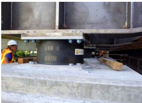
Isolation bearings in Lommen Bridge design will minimize damage to the bridge during major earthquakes
