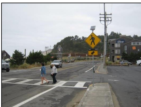
Cape Kiwanda Solar Pedestrian Lights
