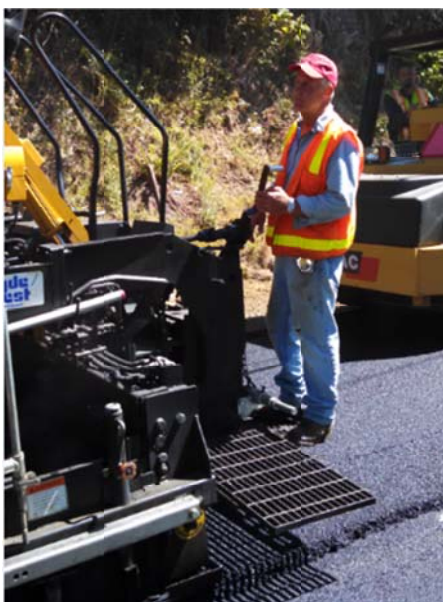
Purchase of a used paver allows the Road Department to repave road sections across the County in FY 2014.
