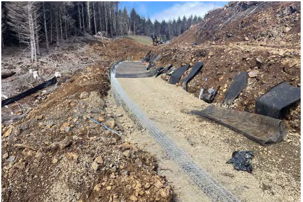
View of the start of the fifth course on MSE Wall No. 2.
