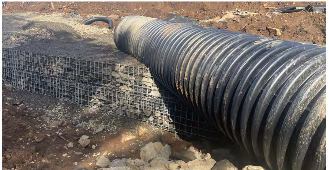
View of initial segment of 36-inch culvert placed within MSE Wall No. 2.
