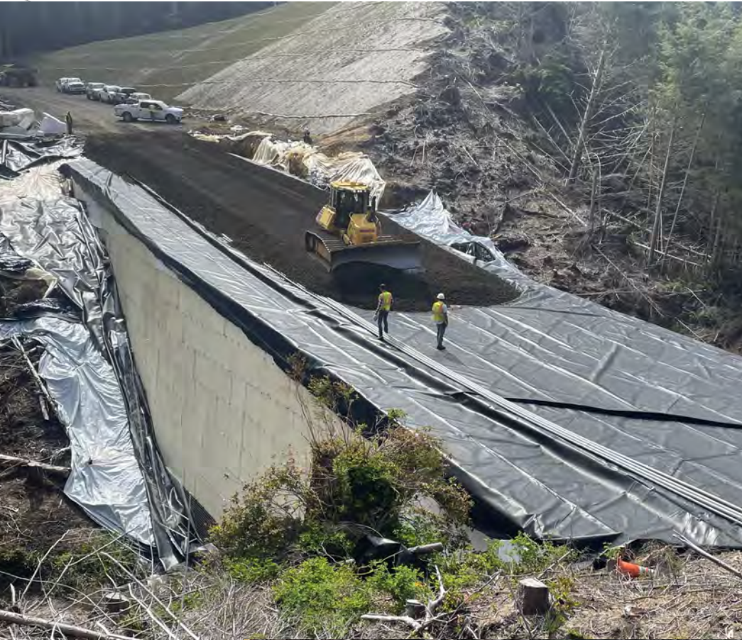
View of geofram wall showing protective membrane and initial lift of roadway base aggregate.
