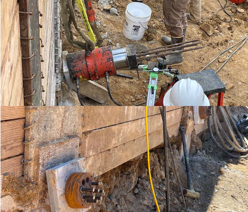
View of ground anchor during stress testing (top) and after final lock-off (bottom).
