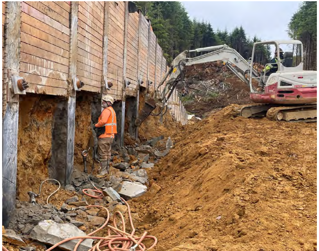
View of excavation at the soldier pile wall in order to extend the height of the wall downward.
