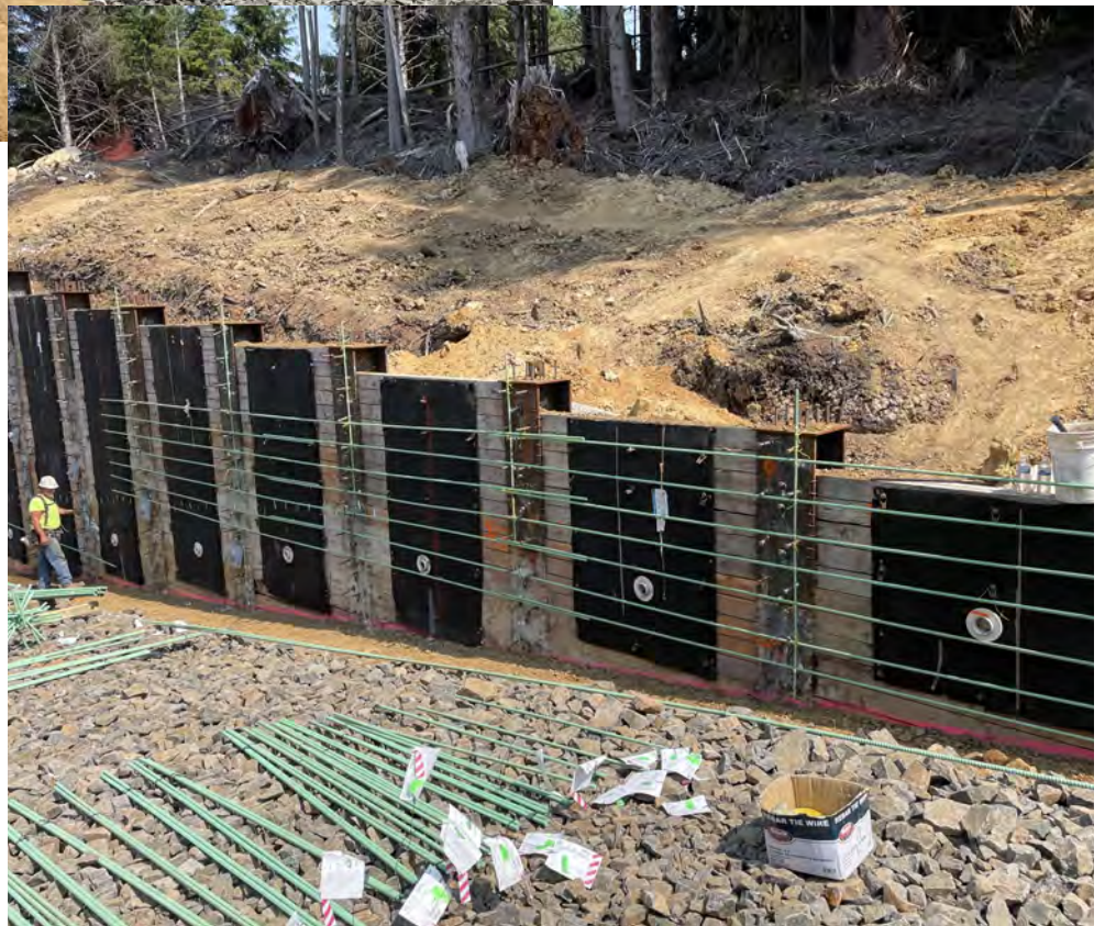
View of first reinforcing steel bars placed within concrete fascia at the soldier pile wall.
