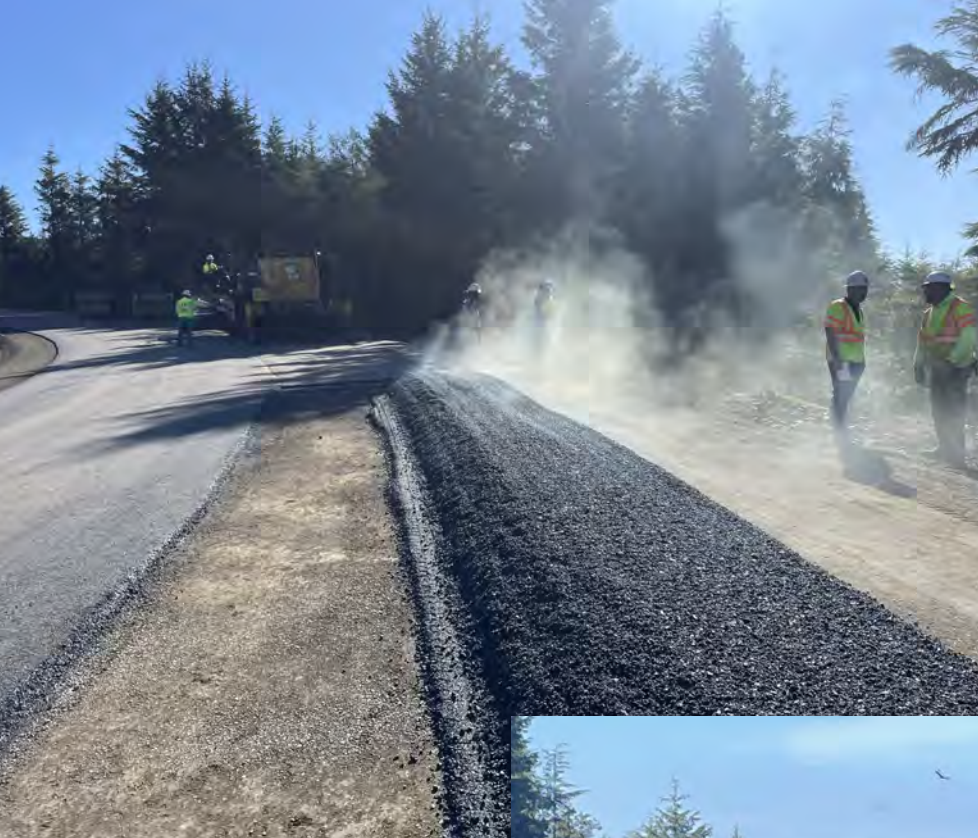
View of freshly placed asphalt ready to be picked up by the paver and evenly spread across the lane.
