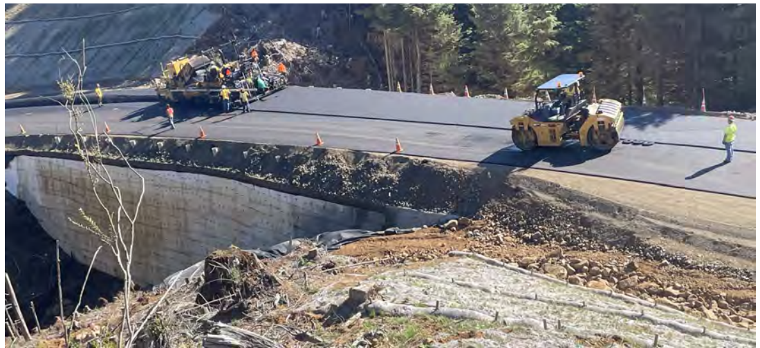
View of top lift of asphalt being placed over the geofoam wall.
