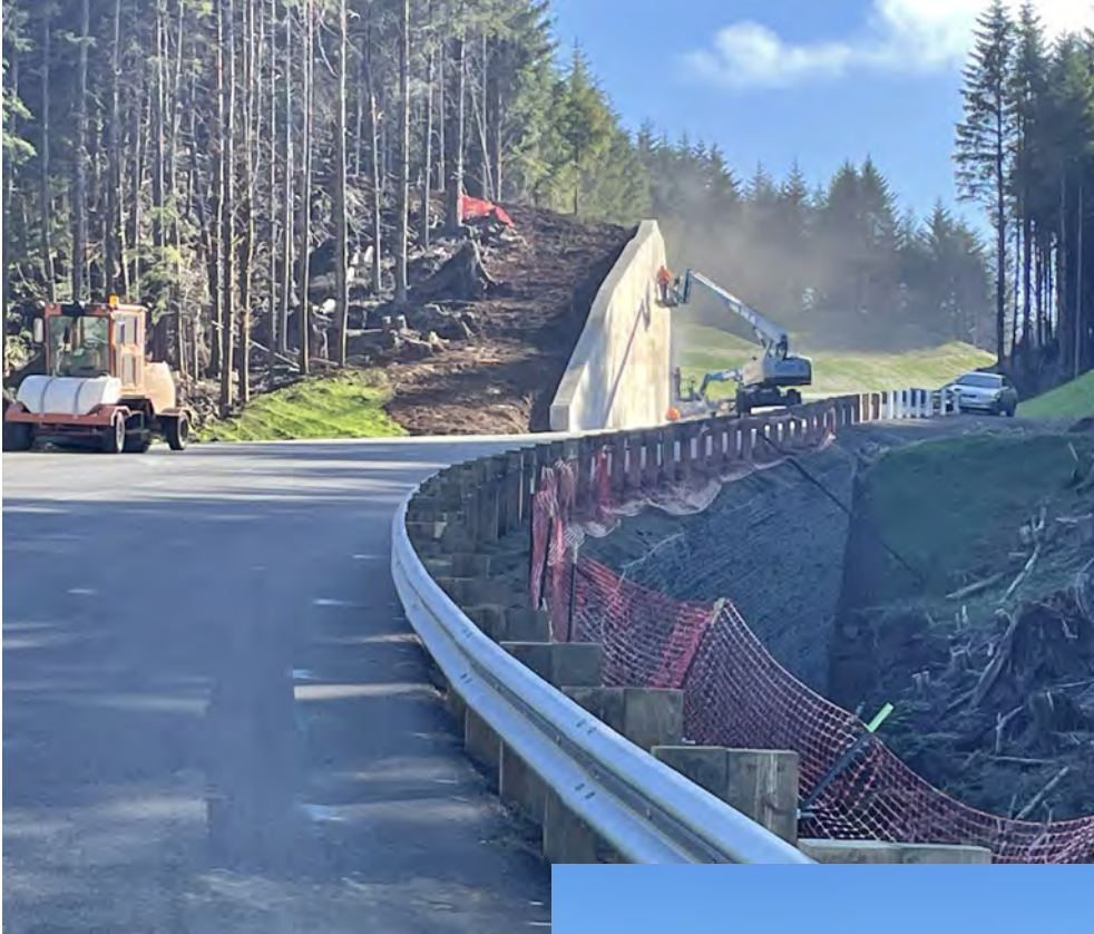
View of completed guardrail at MSE Wall No. 1 with Soldier Pile Wall shown in the background.
