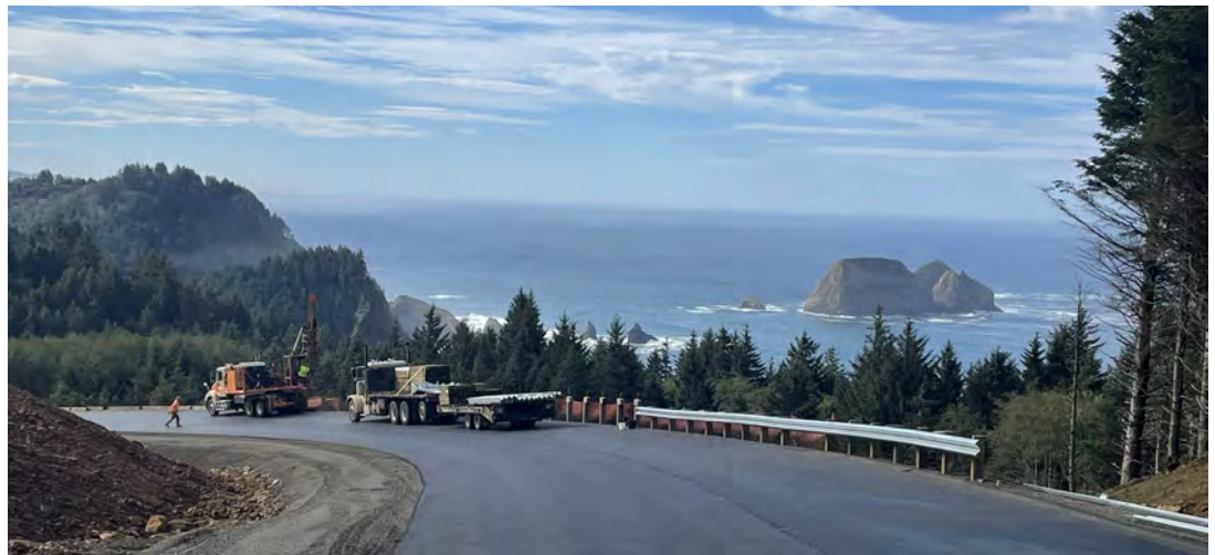
View of guardrail installation at MSE Wall No. 2 overlooking Three Arch Rocks.
